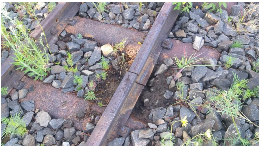
Some of the many rail joints with missing fish plates on the mountain section.
