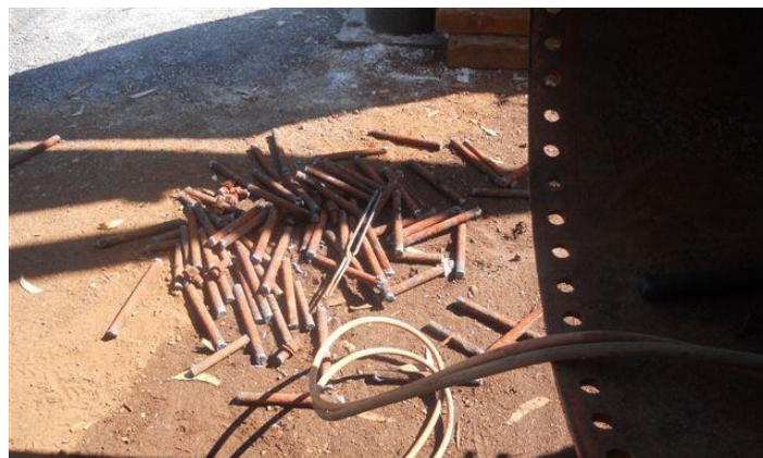
The crown stays after being cut off
