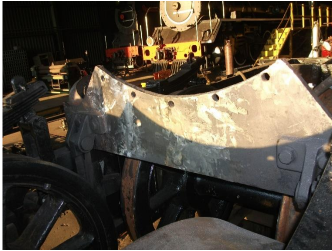
The boiler belly plate.
