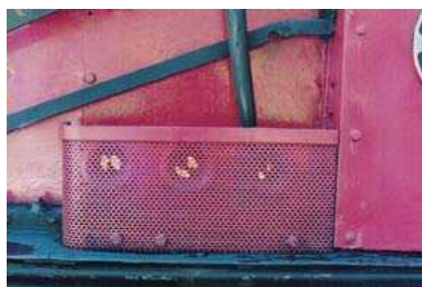
The secondary airvents for the GPCs
