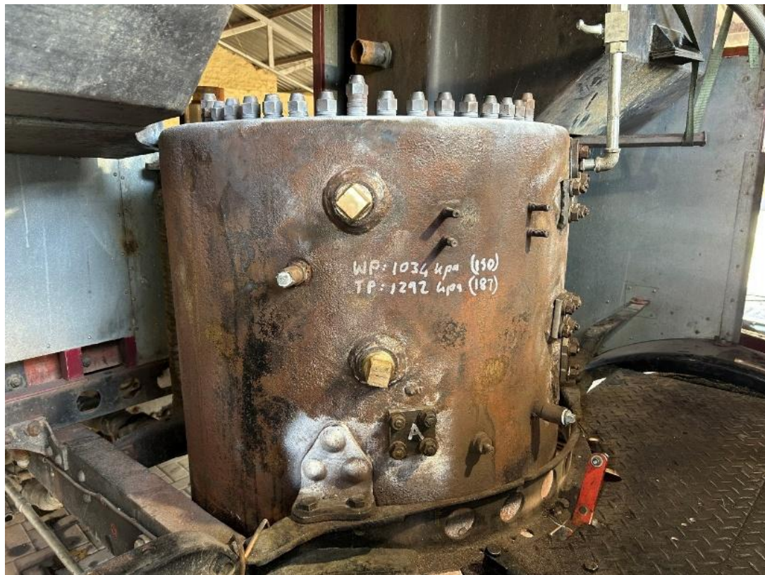
The S4 boiler awaiting its test.
